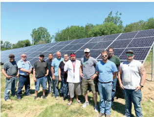
Macy Campus students and contractors working on the installation of the solar panels May 2021
